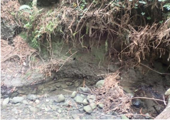
Pomo Creek undercutting its bank. Note the exposed tree roots.
